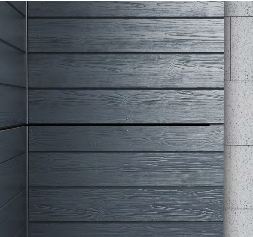
View 2 of clear open joint
